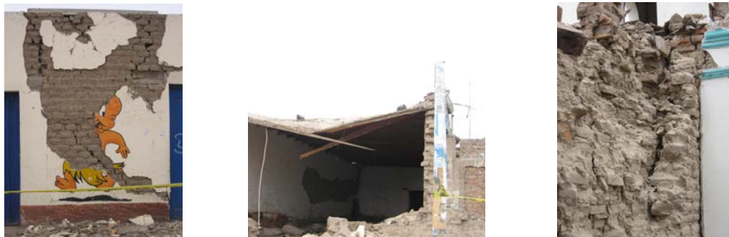
a) In-Plane Damage b) Out-of-Plane Failure c) Wythe Peeling
