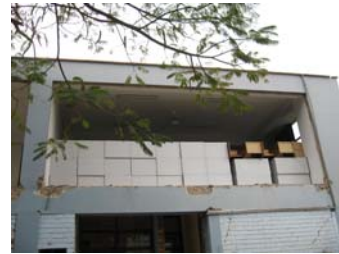
c) Infill Out-of-Plane Collapse
