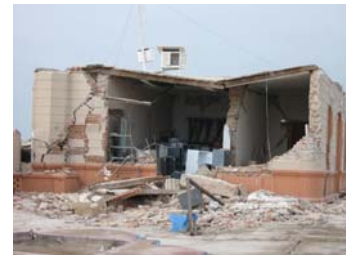
c) Ground Subsidence
