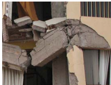
b) Inadequate Transverse RF
