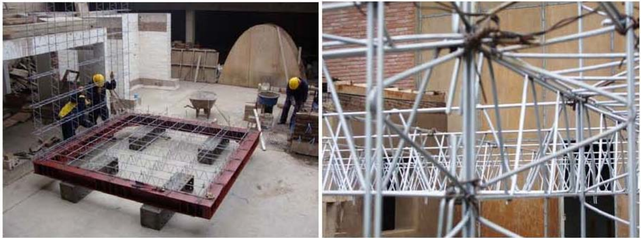
Figure 3: a) Construction of 3 m x 3 m outer ring; b) Wire connection between trusses
