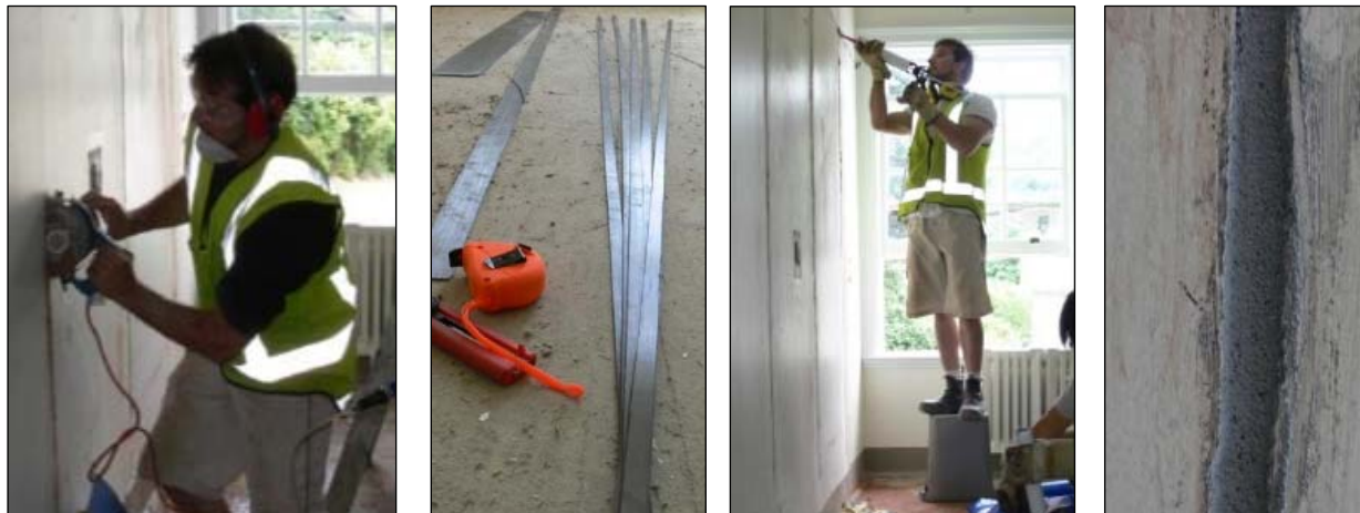
Figure 6: a) Groove cutting b) 15 mm CFRP strips c) Epoxy application d) Groove pointing
