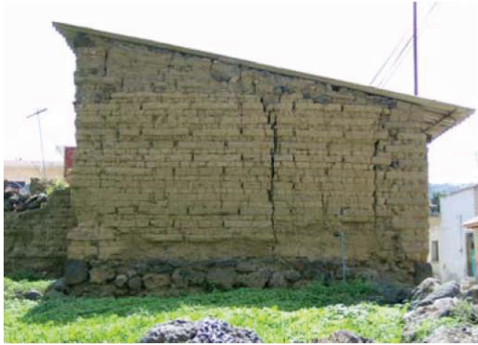
Figure 3: Adobe house in Tlayacapan, presents vertical cracking, there are no beams or columns. A short wall of stones on the base is not sufficient, on support the house on foot. Its roof is laminate.
