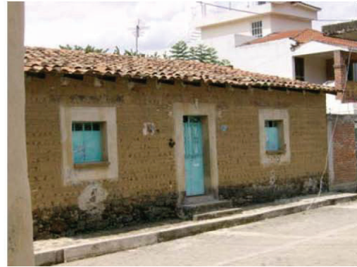
Figure 4: Another adobe house with reinforcements. See the frames on doors and windows and on its base with stones about 50 cm high. The roof is with tiles.
