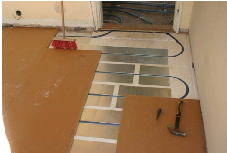
Fig 4. Floor heating system. Circulating hot water on all floors, except natural stone. Pipes buried in polystyrene foam or in concrete on foam
