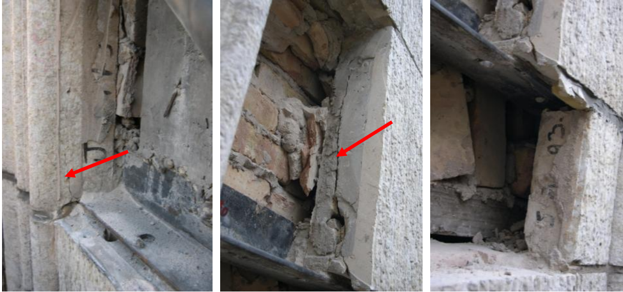
Figure 9: Representative distress in terra cotta at shelf angle locations.
