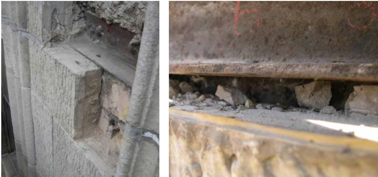
Figure 8: Representative examples of shelf angle locations with minimum bearing (left) and with expansion joint having been cut below shelf angle (right).
