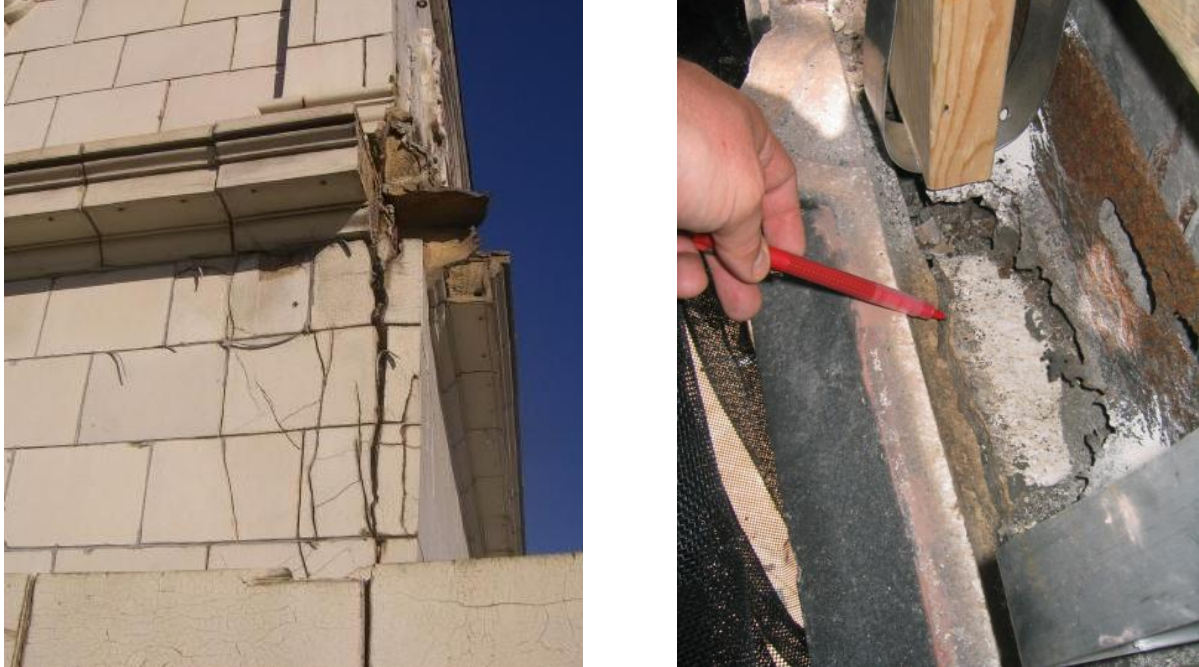
Figure 2: Representative examples of extreme deterioration due to improper maintenance.
