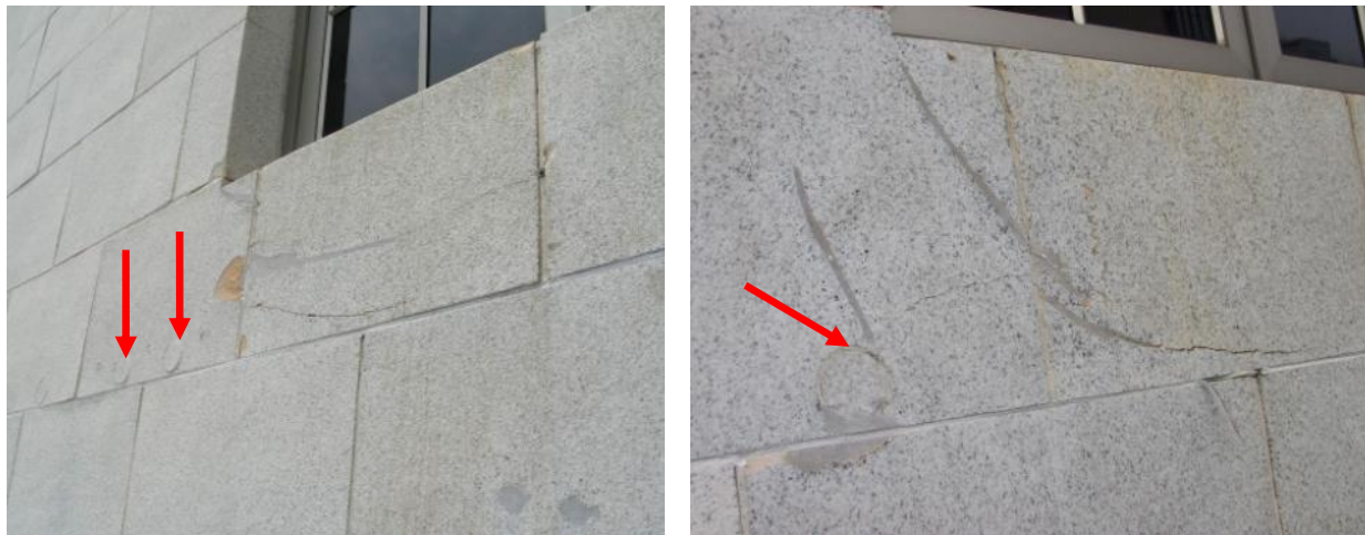
Figure 6: Representative distress in terra cotta. Note locations of previous repairs (arrow)
