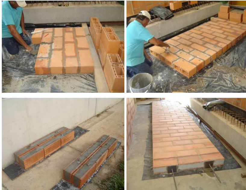
Figure 9: Panel building process 2 – the entire panel is built by laying blocks horizontally
