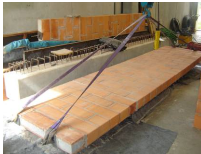
Figure 10: View of the completed panel – the element is suspended by its ends
