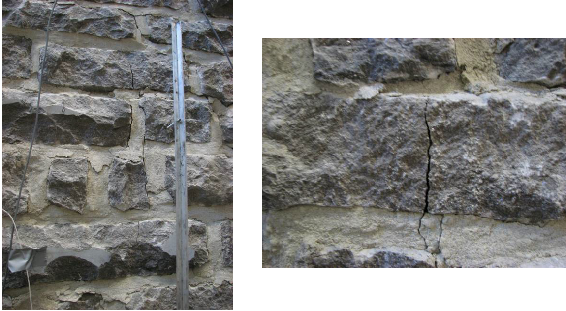
Figure 7: The cracking on the lime stone face (left), and a close up of a cracked limestone
