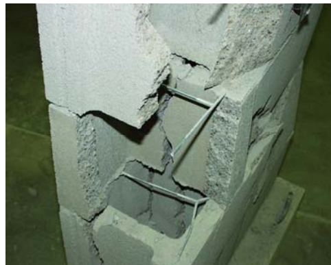
Figure 6: Observed deformation of the joint reinforcement.
