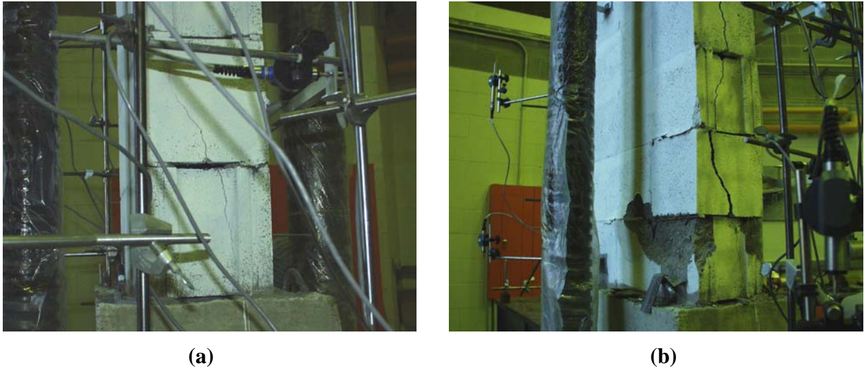
Figure 5: Typical wall crack patterns: (a) Initial cracking in end web; and (b) Tensile-compressive cracking and spalling at ultimate conditions.
