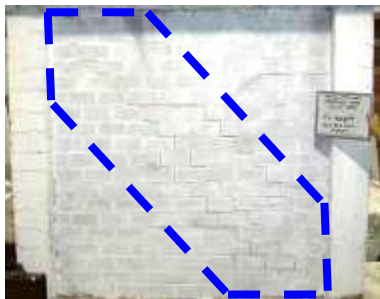
a) Diagonal Crack Patterns at Drift 0.77%
