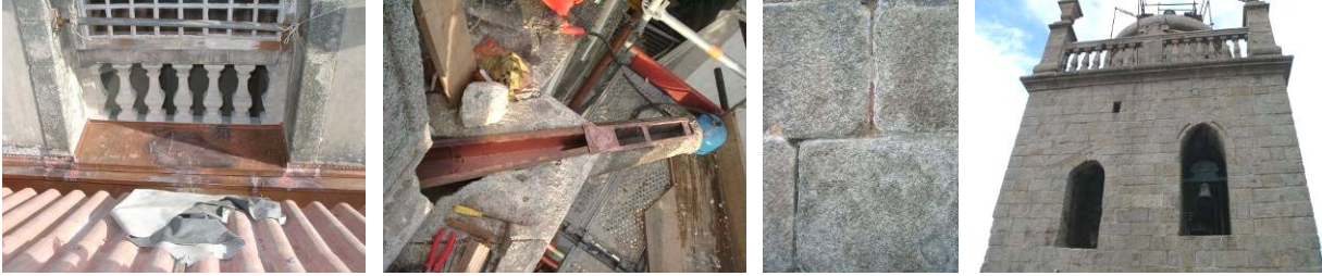
Figure 5: Keeping the Water Out, with Protection of the Granite Stone by Copper Sheeting in External Horizontal Planes and Repointing Joints with Lime Mortar.
