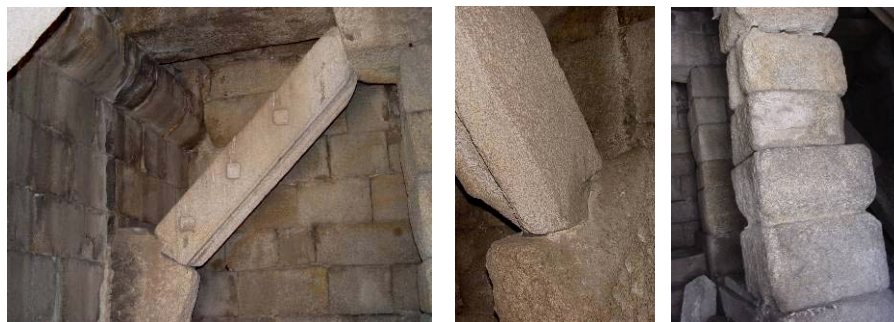
Figure 11: Deficient Structural System to Support the Bell Stone Level Floor.
