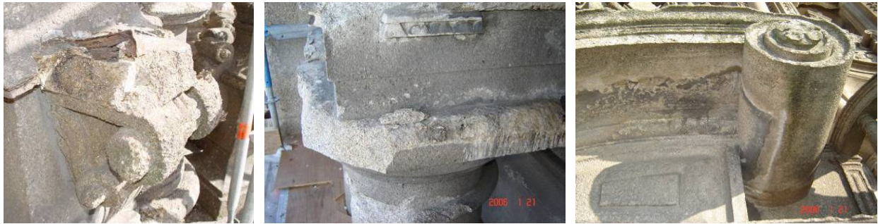
Figure 26: Examples of Stone and Iron Deterioration.
