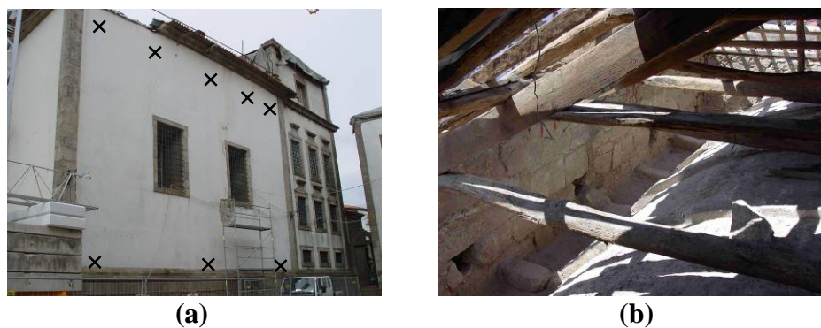
Figure 16: Infill Removal: (a) Location of Topographic Targets for Monitoring; (b) Aspect of the Cleaned Vault.
