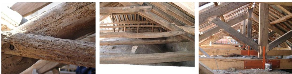
Figure 2: Works in Roof Structures Included Cleaning, Application of Biocide, Application of Preservation Products, Consolidation, Strengthening and Local Replacement. Other Experts Were Responsible for Diagnosis and Specific Treatments.
