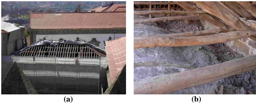
Figure 14: Roof of Saint Vincent Chapel: (a) Aspect of Restoration Works; (b) Aspect of Vault Infill with Rubble.
