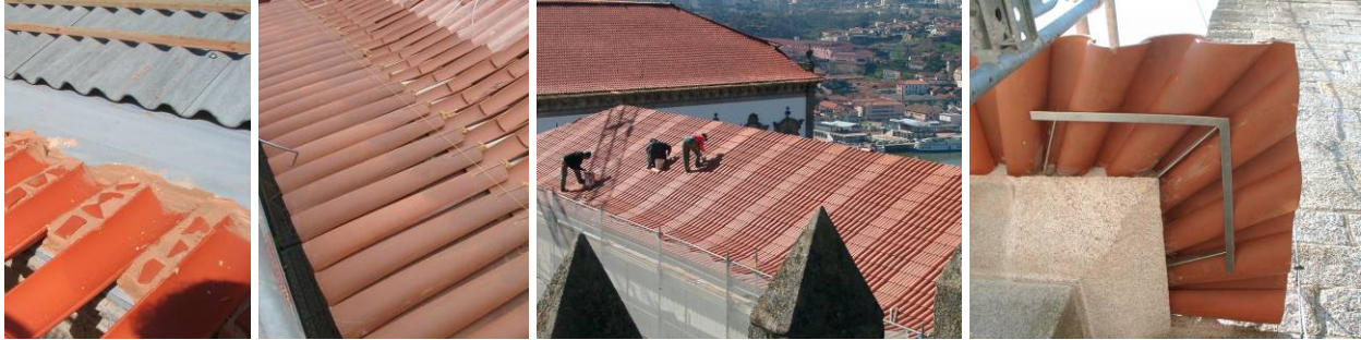
Figure 3: Replacement of the Ceramic Tiles Including New Anchors, Traditional Eaves, Strengthening in the Corners, and Introduction of Sheeting and Walkways.
