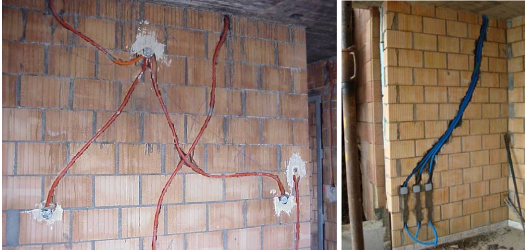
Figure 1: Arbitrarily Cut Chases in Masonry Walls
