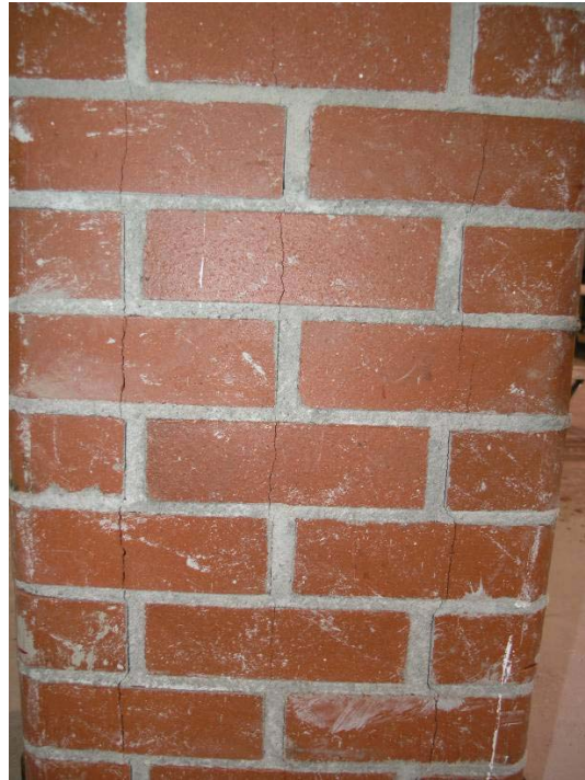
Figure 4 – Cracking in a plain column
