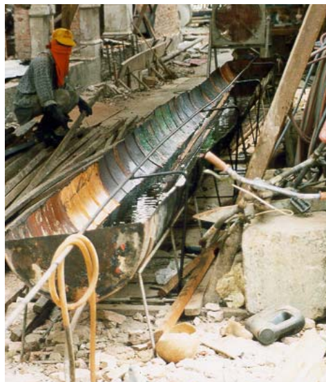
Figure 11 – Trough Used for Termite Protection
