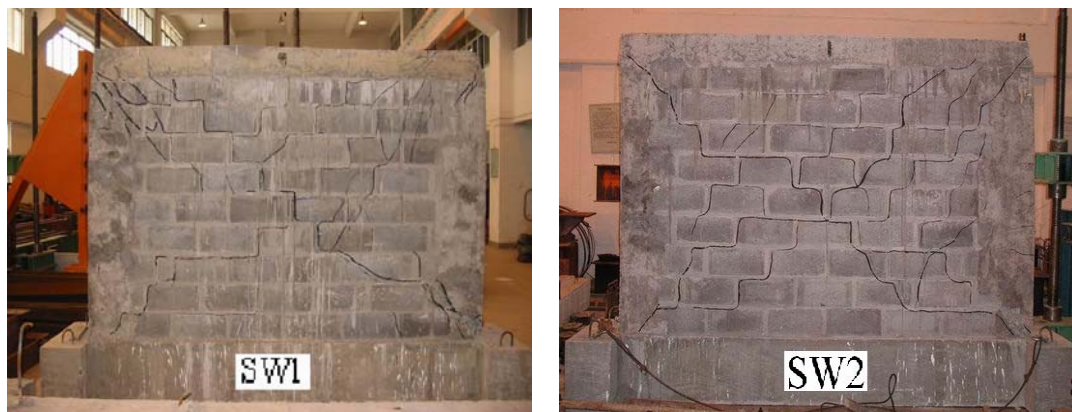
Figure 3 – Failure Patterns of Walls
