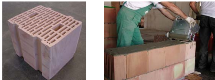
Figure 1 – Edge-ground units used for the research (TM, left) and construction of a specimen (right)
