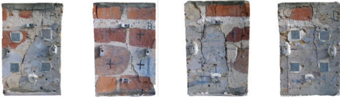
Figure 5 - crack pattern of prism II 12 at the end of test, face A, B, C, D
