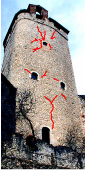
Figure 7 – Avio Castle. Crack pattern of the Mastio
