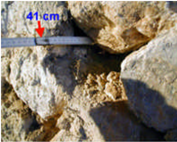
Figure 17 – Direct inspection which indicate the presence of a void
