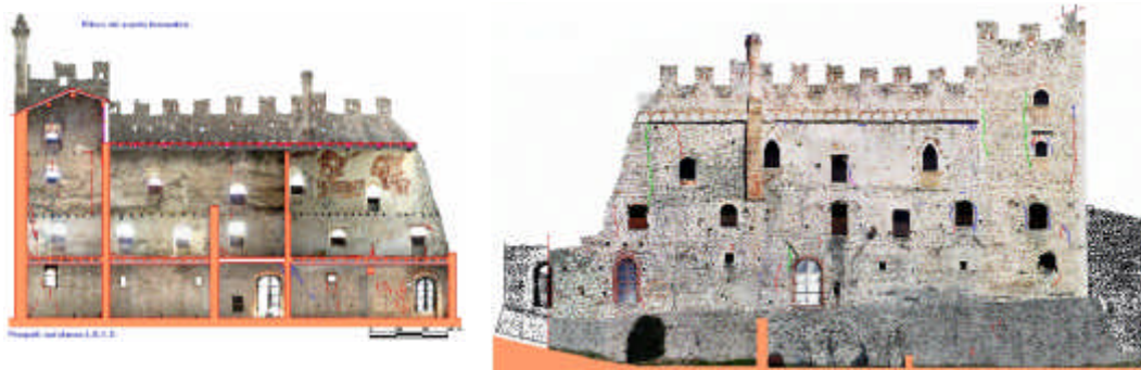
Figure 2 - Avio Castle Crack pattern survey of the South wall
