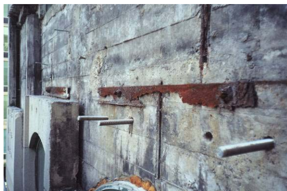
Figure 10 – 15 th floor stones removed. 3 previous retrofit anchors and an extremely corroded original shelf angle shown.
