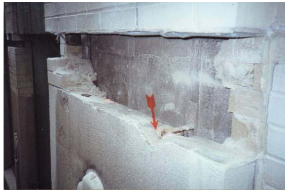
Figure 9 – Typical Spall (red arrow) at Corroding Lateral Stone Connection (brick has been removed from above stone).
