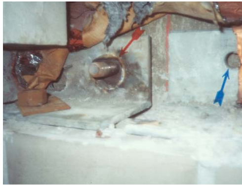
Figure 7 – Shelf Angle Deficiencies Include Missing Anchor (Blue Arrow), Oversize Burnt Hole (Red Arrow), and Lack of Soft Joint Below Angle.
