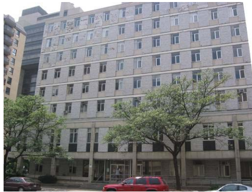
Figure 1 – East Elevation; Extensive Spalling Of Glazed Bricks
