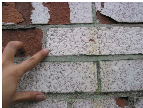
Figure 2 – Close-Up of Glazed Brick Spalls
