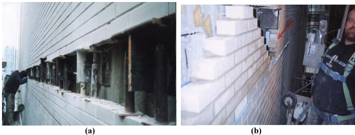
Figure 6 – (a) Temporary Masonry Post Shores in Place while the Inverted Angle Brackets are being Installed; (b) Masonry Being Reinstalled in Sections After the New Shelf Angle has been Installed
