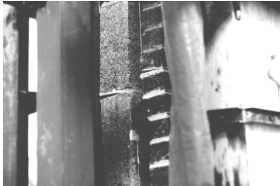
Figure 6: Mid-height bed joint separation
