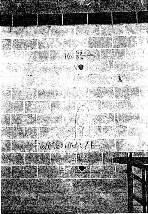
Fig. 7 — Verification of impact-echo testing.
