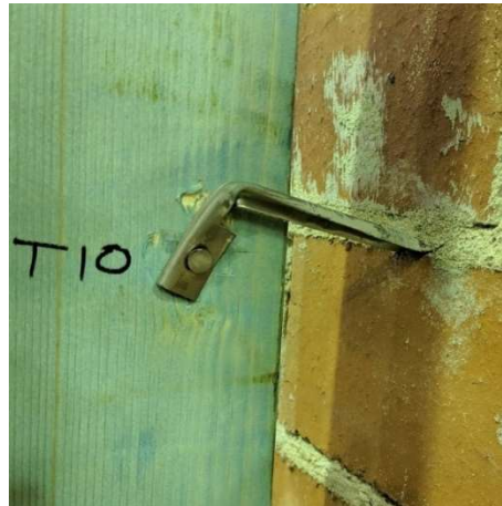
Figure 11: Typical (Buckling) Tie Failure Observed in Veneer Wall Tests
