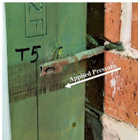
Figure 12: Nail Pull Out Tie Failure Observed in Veneer Wall Tests
