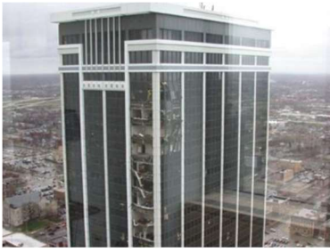
Figure 5: One Indiana Square. Wind damage from microburst wind event.
