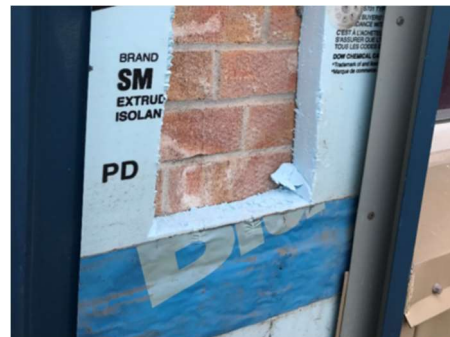
Figure 7: St. Clair Birchmount I. Probe in existing rainscreen overcladding revealed insulation added to increase the thermal performance of the building.
