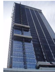
Figure 7: One Indiana Square, Indianapolis, IN. Overcladding installation performed from mast climbing scaffold.
