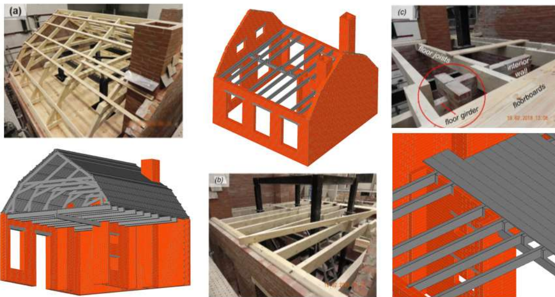
Figure 3: Photos of a) roof and b) first floor of LNEC-BUILD-3 during construction [21] and related numerical model views
