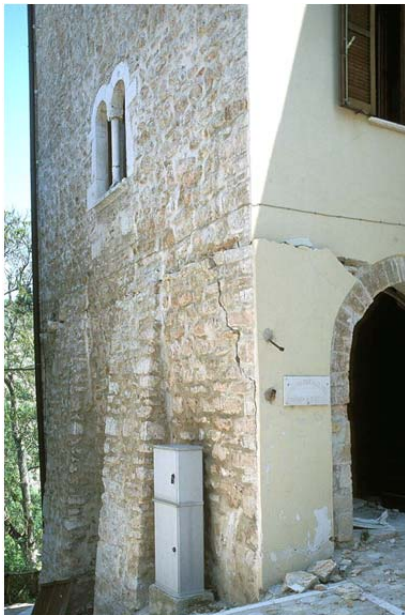
Figure 6: Rigid R.C. Sheared and Delaminated Stone Masonry Walls at Supports [10]
