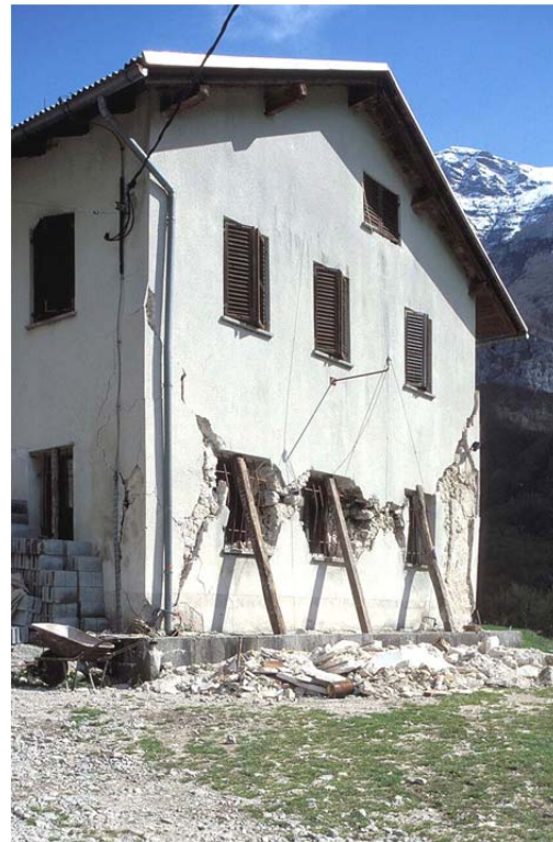
Figure 2: Shear Failure of Walls
