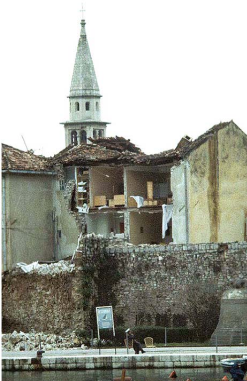
Figure 1: Out-of-plane Collapse of Walls
