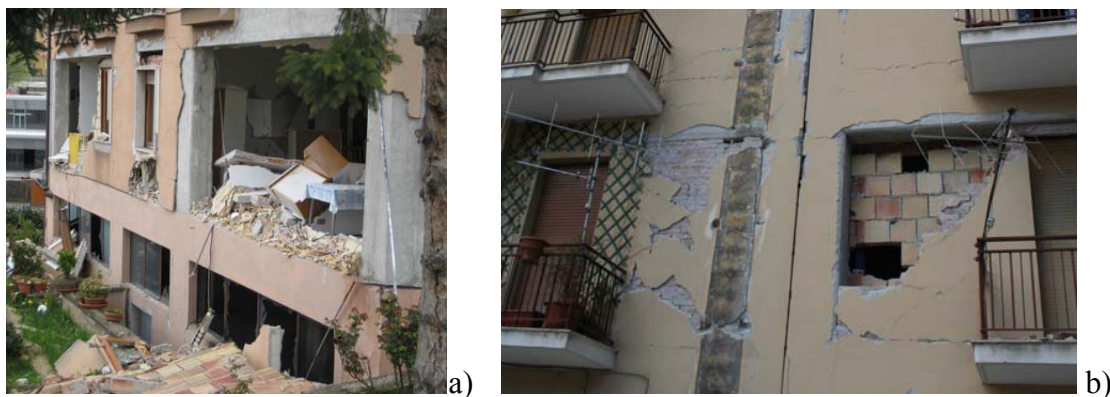
Figure 1: Out-of-plane collapse of infill walls in r.c. framed structures registered in the regions struck by recent earthquakes in Italy [7]
