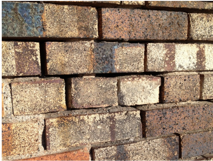
Photo 2: Kiln #1- A typical example of deteriorated mortar joints
