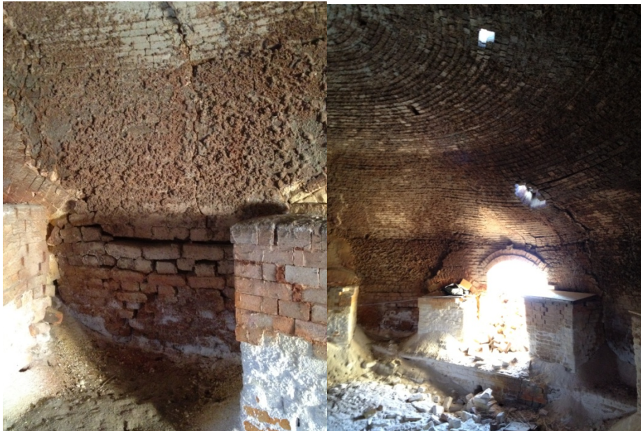
Photo 7: Kiln #6- Interior deflection of the walls and dome
