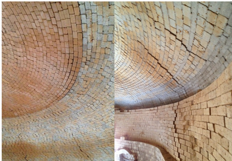
Photo 5: Kiln #9- Horizontal cracks half way up the dome and Deflection at the base of the dome
