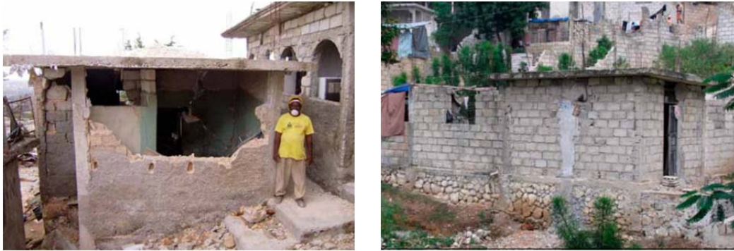
Figure 1: Earthquake destruction in masonry houses in Haiti [2]: a) Out of plane failure; b) Lack of column at corner
