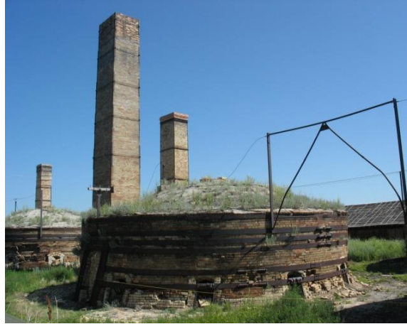
Figure 4: Example of abandoned kiln as example of advanced deterioration showing foundation settlement, mortar and masonry deterioration and biological growth.
