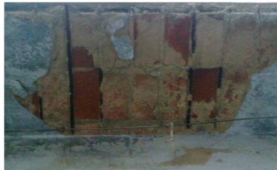
Figure 2: Deterioration of RB slabs
