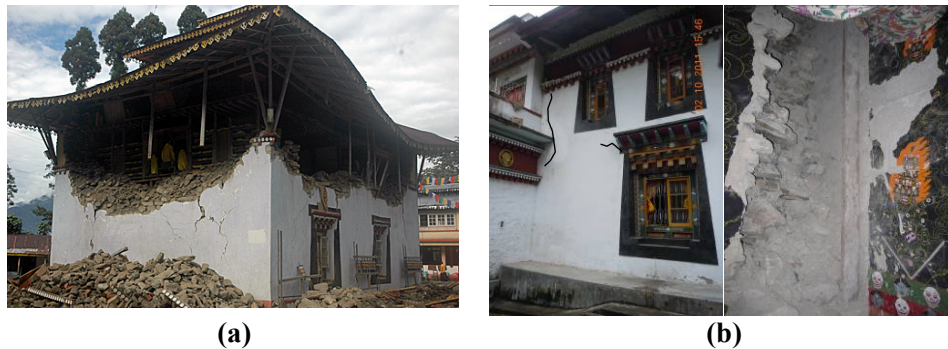
Figure 4: Common damages observed (a) Partial collapse of wall of Ringhem Choling monastery and (b) Shear cracks and delaminated wall painting at Samten Choling monastery.
