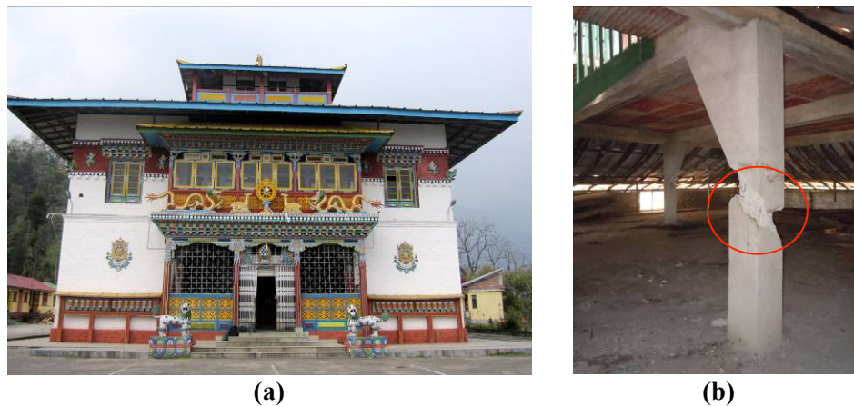
Figure 7: (a) Phodong monastery, interior RC frame with exterior stone masonry wall and (b) Damaged column due to short-column effect induced by the presence of deep haunches
