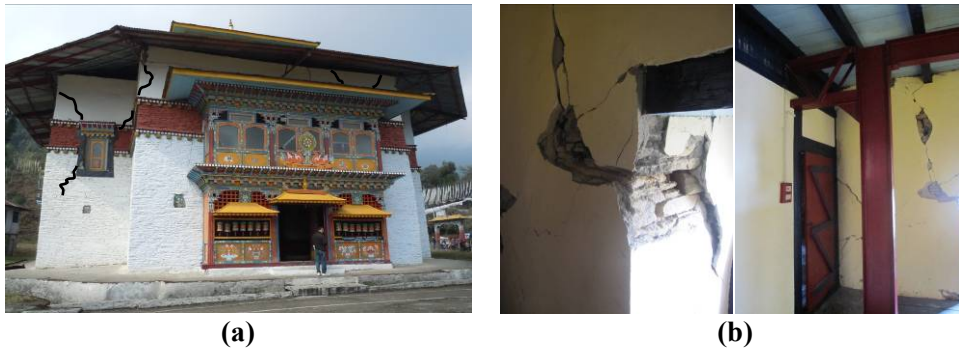
Figure 6: (a) Cracks on the exterior wall of Labrang monastery and (b) Exposed stone laminates during the recent damage and steel columns and joists used in the retrofit
