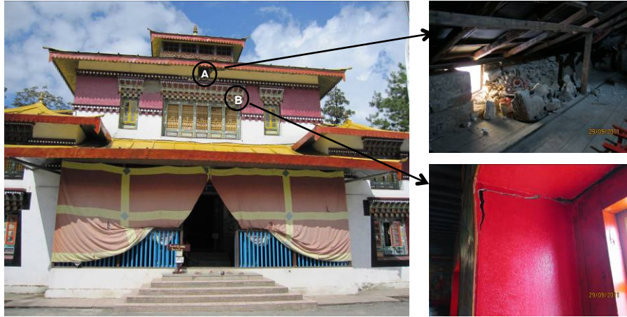
Figure 5: Damages observed on the front wall of third storey at Enchey monastery
