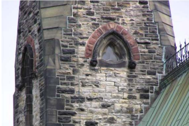
Figure 8: A Diagonal Crack in the Tower
