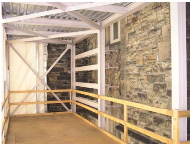
Figure 6: Emergency Stabilization of Wall Bulging
