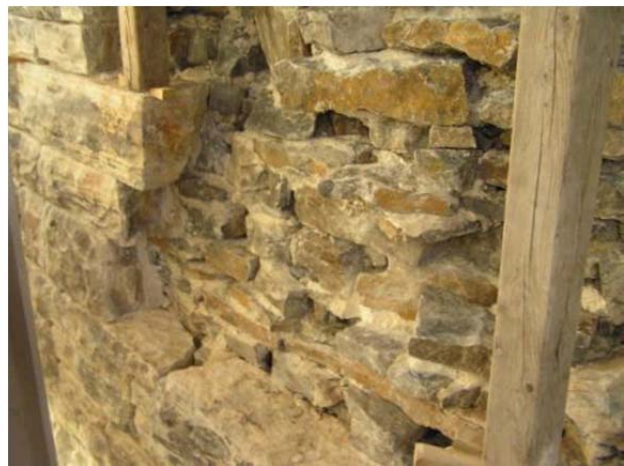
Figure 7: Evidence of Wall Delamination
