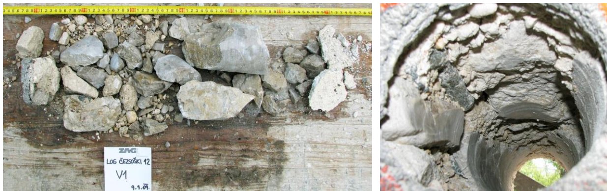
Figure 5: Less effective grouting - the grout is present but didn't connect together the stones and mortar
