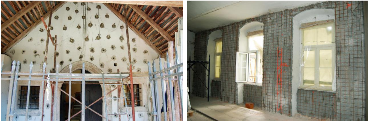
Figure 3: a) Systematic cement-grouting of masonry b) Reinforced cement coating: steel mesh is placed after steel anchors are fixed through the floor structures and adjacent walls.
