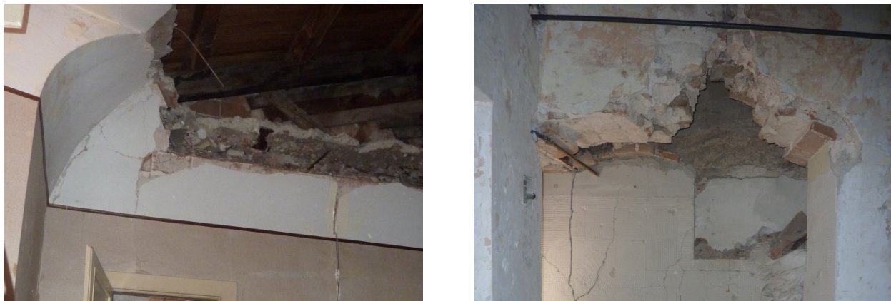
Figure 4: View of damaged vaults and architraves after the earthquake
