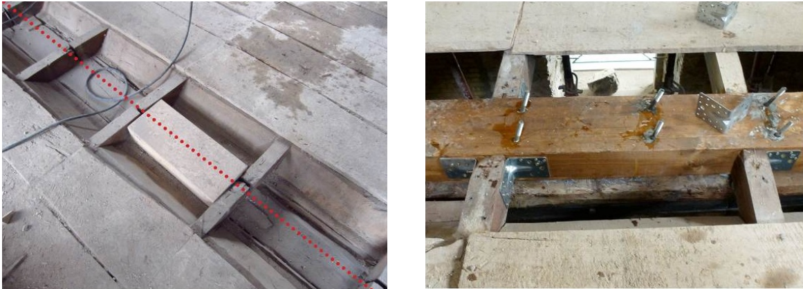
Figure 16: Increasing depth of timber beams with timber blocks and fastening of lintels
