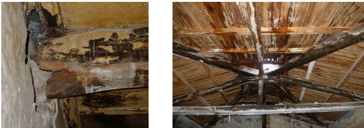
Figure 6: View of timber beams and frames with damaged sections
