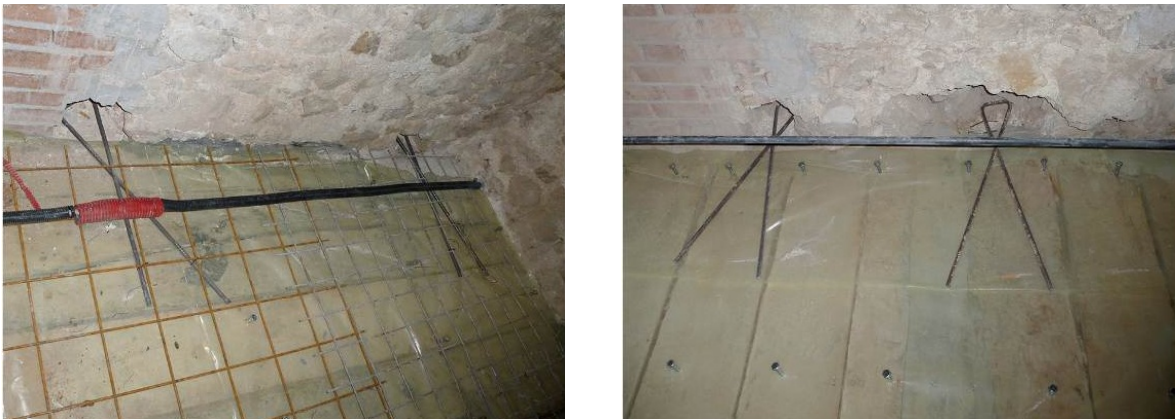
Figure 17: Steel ties placed around rooms and edge connectors to be grouted into the slab
