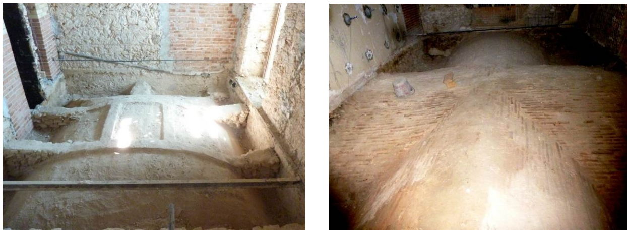
Figure 8: Barrel vault with stone stiffeners and cross vault made with one head bricks
