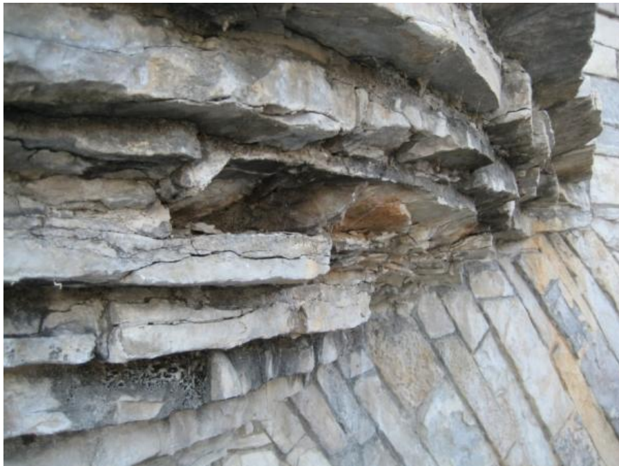
Figure 5: View of Deterioration of Stone at Fountain
