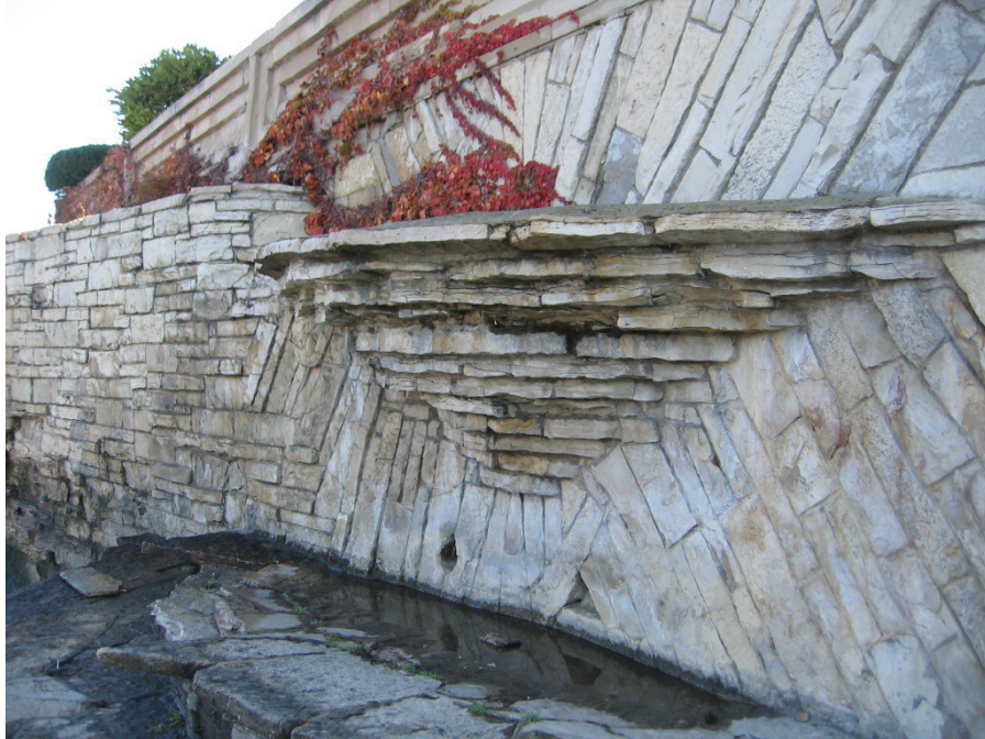
Figure 4: Overall View of Limestone Fountain
