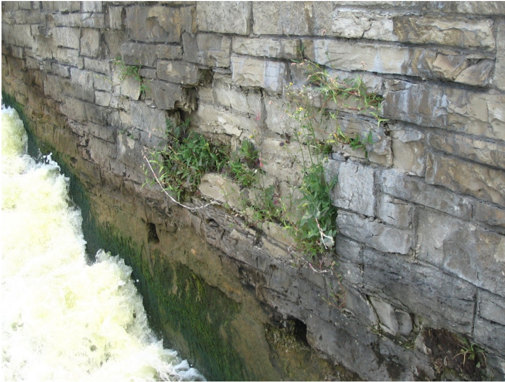
Figure 3: Deteriorated Limestone Adjacent to the Fish Ladder
