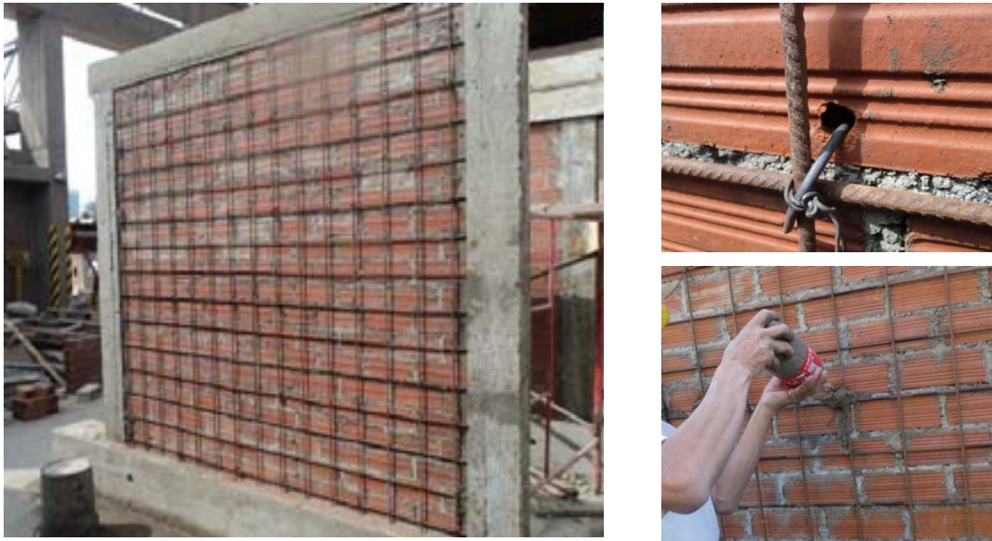
Figure 7: Wire meshes added to W2, detail of connection wire and filling the perforations
