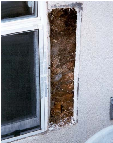
Figure 5. Water Damage Behind Surface Barrier EIFS without a Drainage Plane
