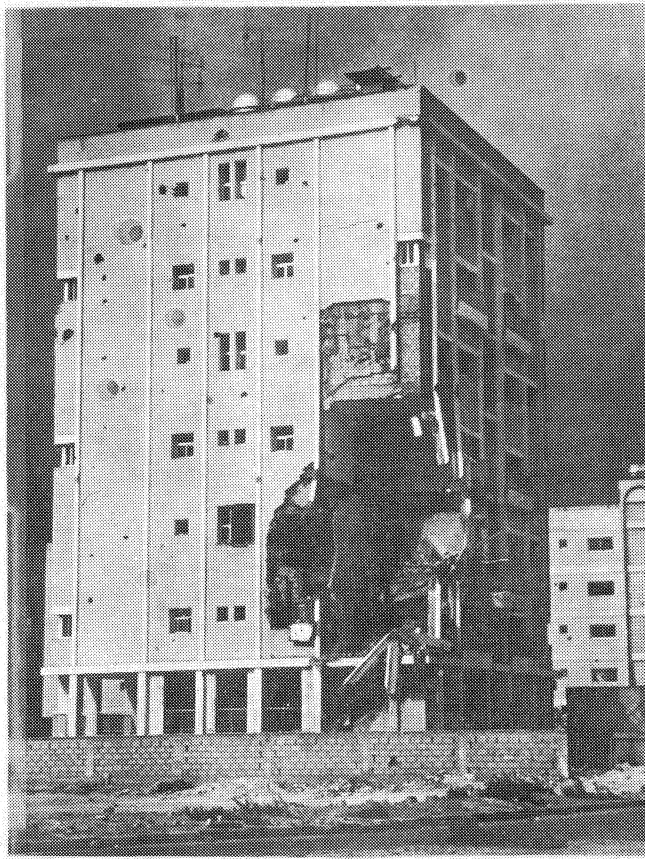
Fig. 3: Building Subjected to Direct Shelling, where the Main Structural Elements Suffered Extensive Damage
