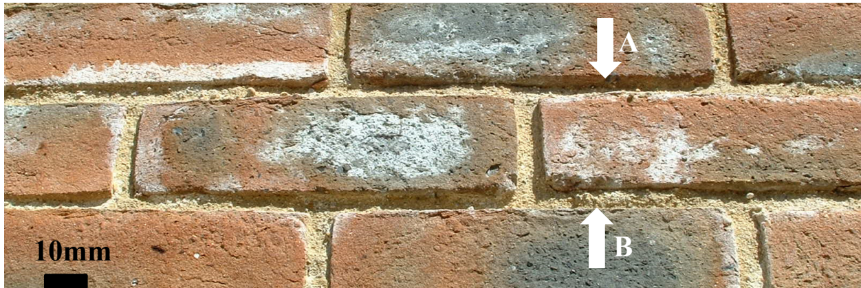
Figure 1: One of the Localised Areas of Brickwork where the Mortar Joint has Eroded Back Approximately 10mm from the Brick Face (A). Blistered and Friable Mortar can be seen in Association with Mortar Joint Surface Efflorescence (B).
