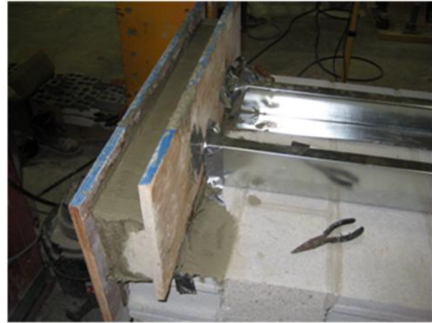
b) Pouring of Concrete Floor to Anchor Reinforcing Tie into the Bottom of the Wall
