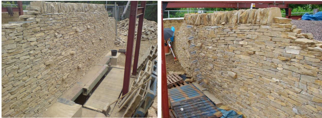
Figure 5: Test wall 1: a) post construction; b) prior to failure
