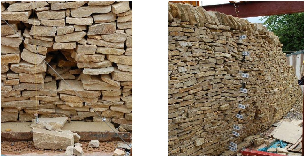
Figure 7: Test wall 3: a) local failure; b) prior to total failure
