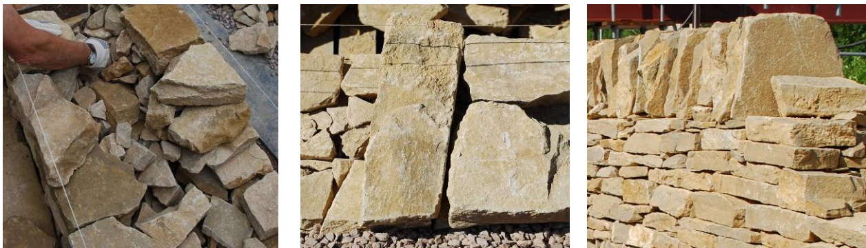
Figure 1: Typical wall details: a) face and fill; b) through stones; c) coping stones
