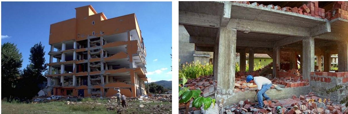
Figure 1: Collapse and Fall of Masonry Enclosures Due to an Earthquake
