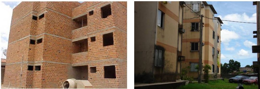
Figure 1: “Caixão” building: a) Building under construction; b) Typical building of four floors, in which non-structural ceramic blocks were used for structural ends.
