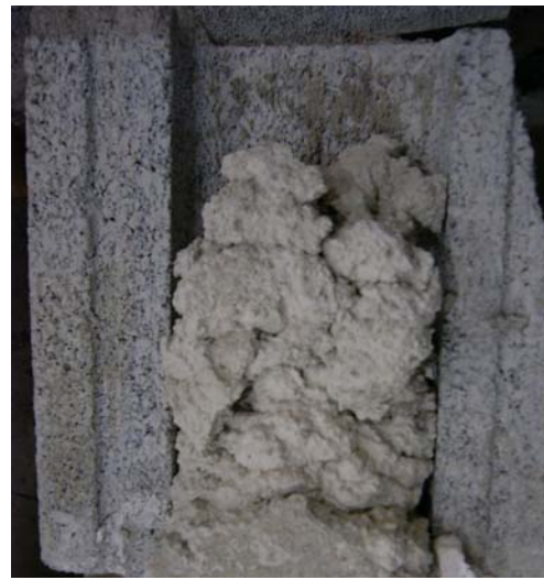
b) Poorly compacted grout
