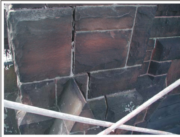
Figure 1 - Evidence of considerable lateral movement within buttresses.
