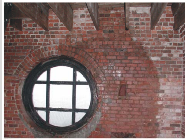
Figure 5 - Evidence of moisture saturation on the interior.
