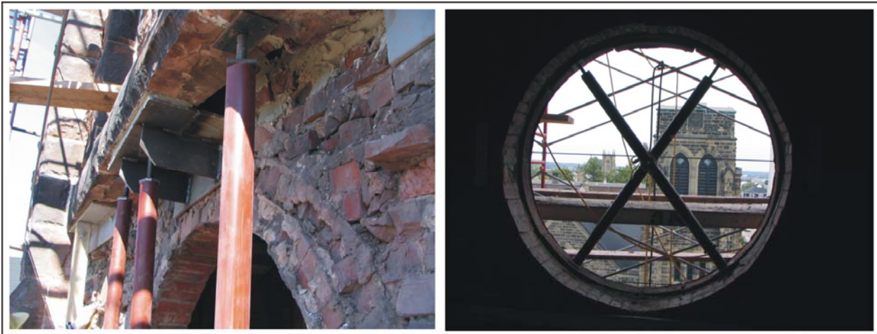
Figure 19 - Examples of temporary and permanent shoring used to support the overhead masonry during masonry rebuilding work.
