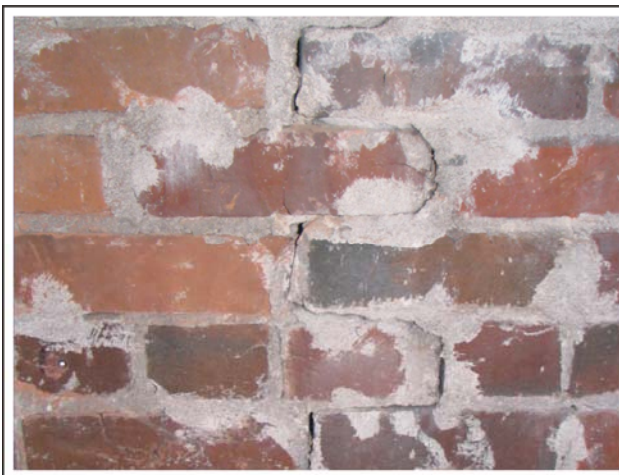
Figure 3 - A step crack within the interior aligned with the exterior buttress joint.
