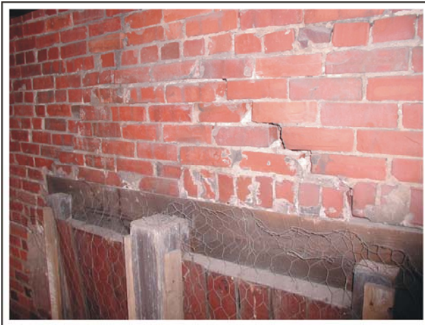
Figure 7 - Evidence of an inward lateral thrust of the masonry.
