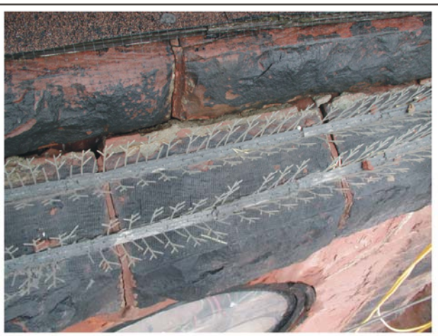
Figure 4 - Evidence of water penetration at several locations.
