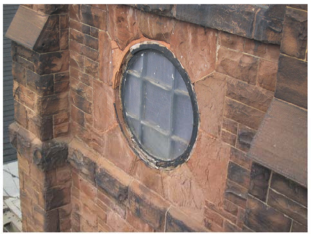
Figure 6 - Evidence of contour scaling and damage to voussoir stones.
