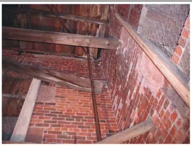
Figure 8 - Evidence of deterioration to one of the wooden floor assemblies.
