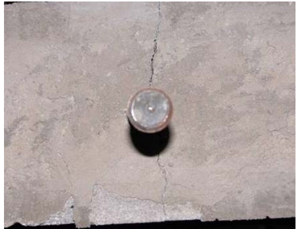
Figure 5 – Onset of Splitting Cracks in Specimen Set A
