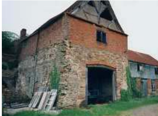
Figure 4 – Missing Nogging in Gable End
