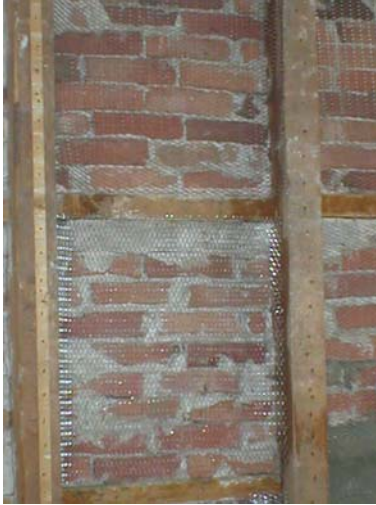
Figure 10 – Brick Nogging with Mesh Attached to Studs
