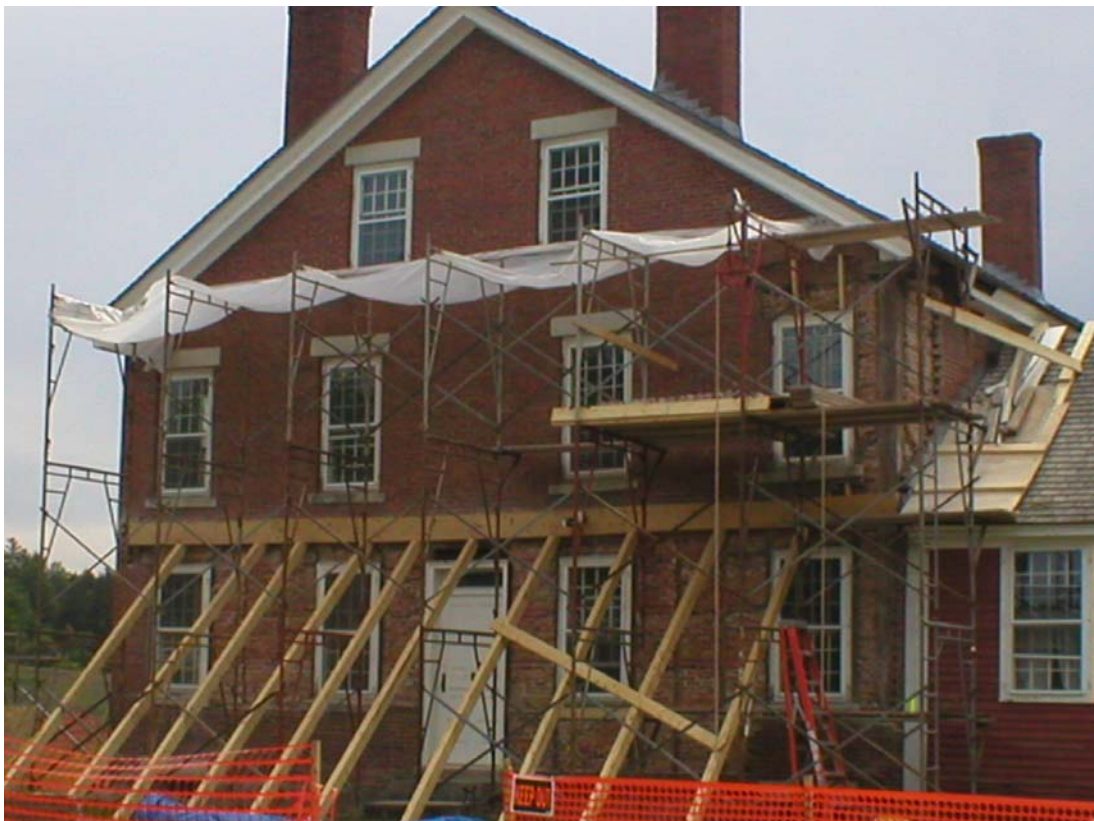
Figure 12 – West Wall with Shoring in Place Veneer Removed Below the Shoring.
